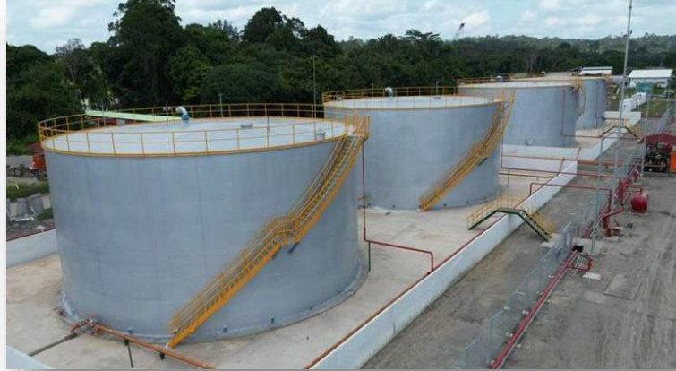
Fuel Storage Tank
