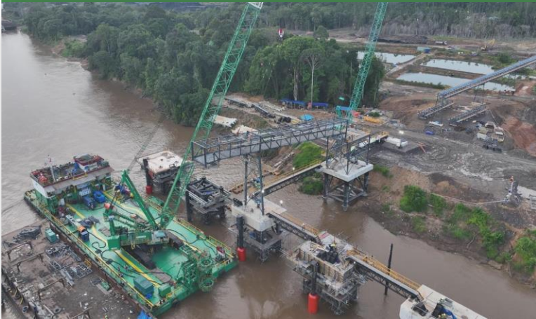
Second Barge Loading Conveyor
